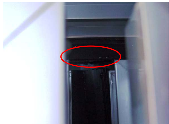
Fig. 16 External coupling gasket not bonded at T-joint
