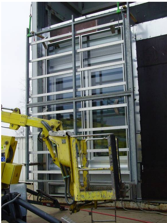
Fig. 3 Facade with water spray grid
